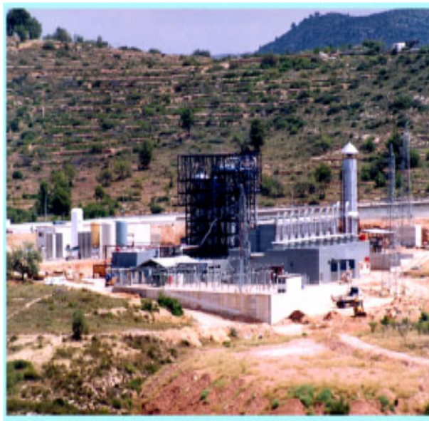
Gasification plant, Castellon, Spain (25 ktpa, 7MWe)
